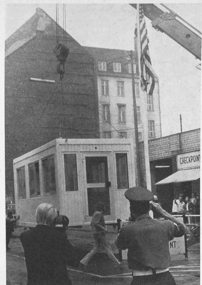
MAY, 1976 — Workmen demolished the building and a brand new "Checkpoint Charlie" came into being. (Photo by Ralph Yoder)
